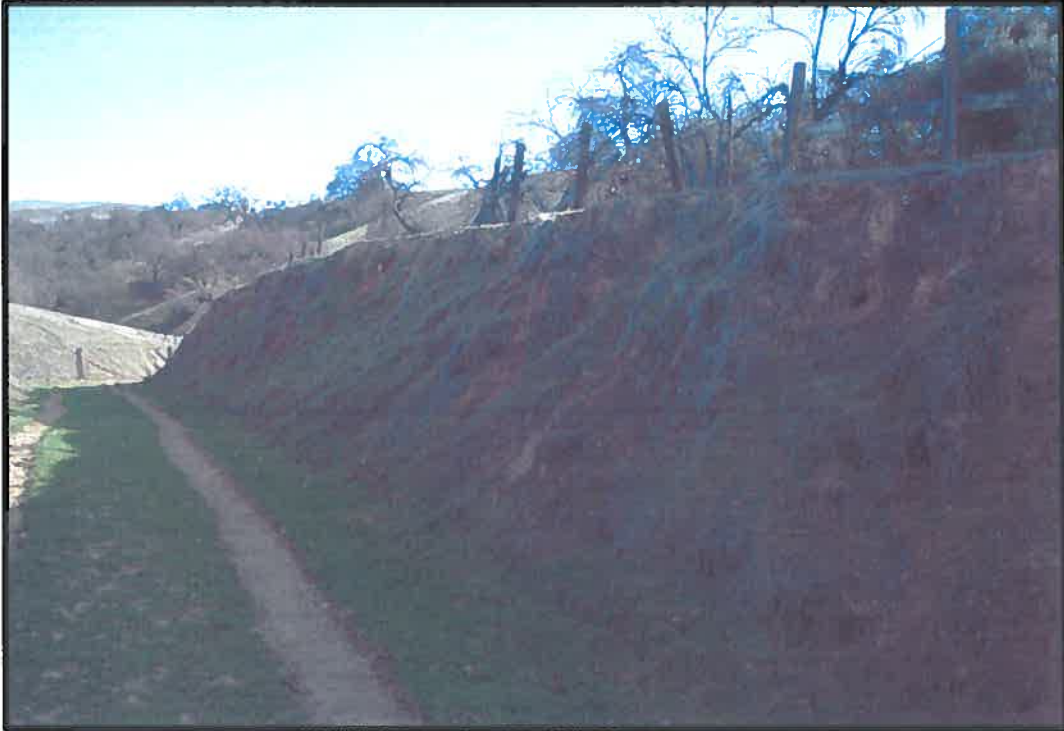
Figure 6: Cut Slope which Exceeds a 25-Percent Grade.
